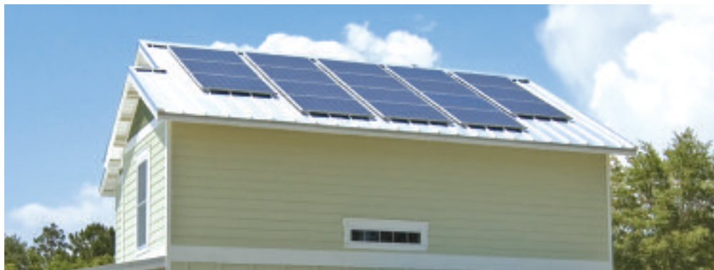
Solar panels on LEED Platinum home help make it "net zero"—so the homeowner can sell back to the power company as much energy as the home uses.
